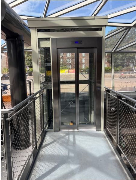
This is the lift from the entrance to the Dry Berth
